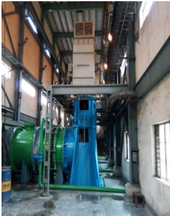
Fig.1. Vertical ACW pump at KSTPS (Unit-6)
